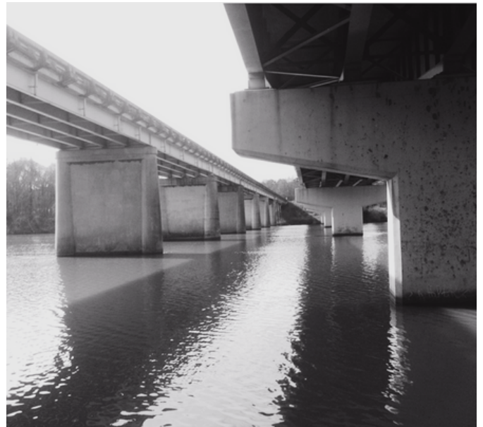
Left Bridge (1924) – First bridge built by F. A. Triplett (Triplett-Small, Inc.) Right Bridge (1976) – Adjacent bridge built by James T. Triplett (JTT, Inc.) SC 9 over the Catawba River Chester/Lancaster County Line, South Carolina
