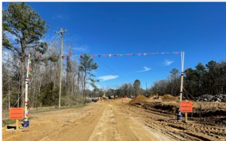
Flagging that was installed at the entrance of Berlin G. Myers Parkway to help warn workers of powerlines.
