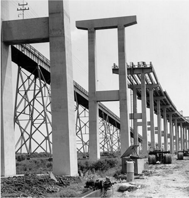
Construction of Silas N. Pearman Bridge in 1965 beside the Grace Memorial Bridge Charleston, South Carolina
