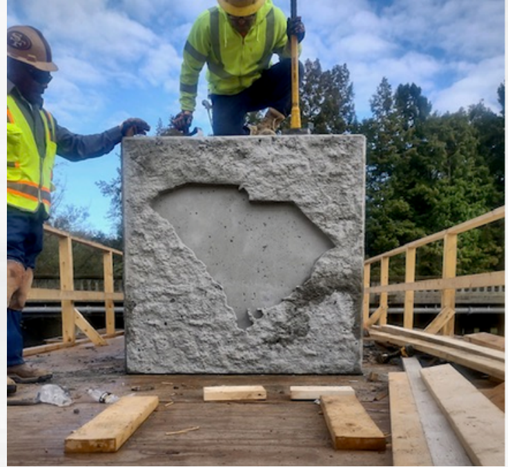
Bobby Edwards, Albert Watts, and their crews poured impressions of SC at the interior caps and will pour Palmetto trees at the end bents.
