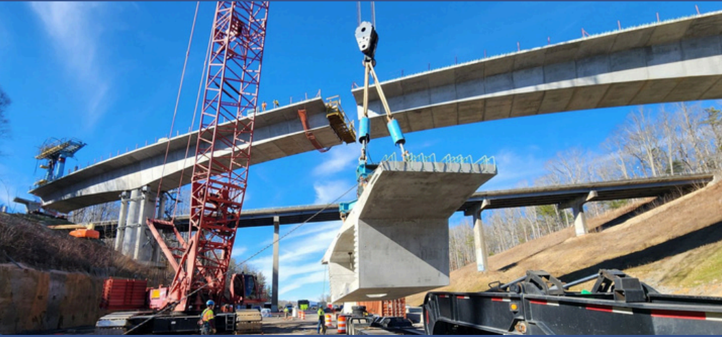
Last segment for Blue Ridge Parkway Bridge over I-26 in Asheville, NC at FUALLC.
